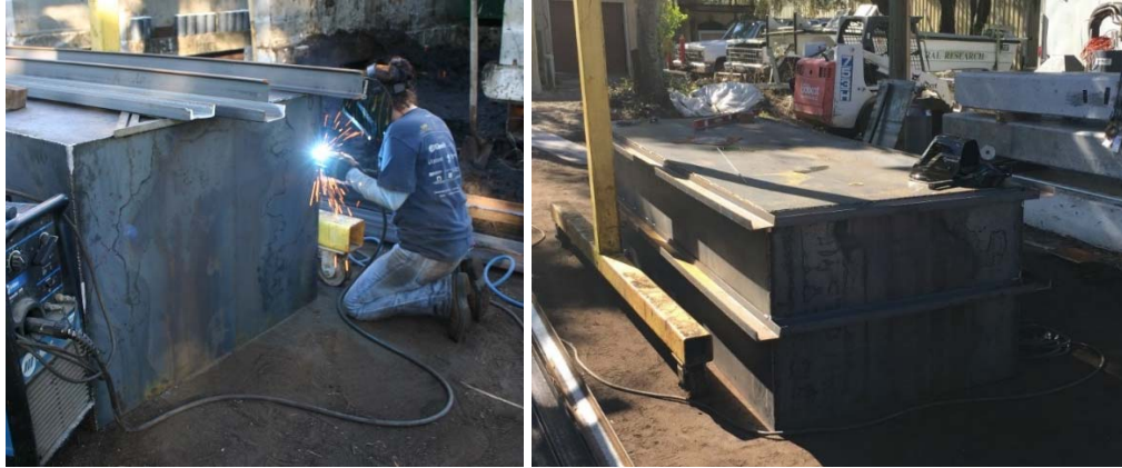
Figure 4.1 Welding of the bed (left) and the bed upside-down during fabrication (right).
