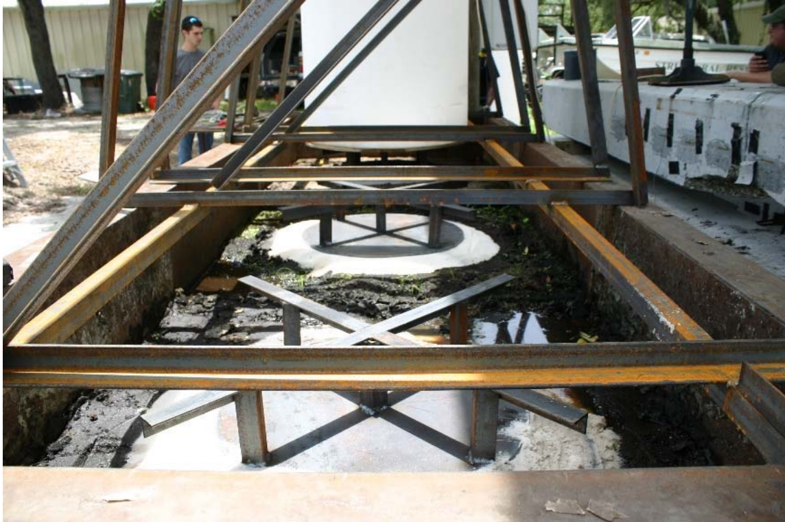
Figure 4.33 Bearing plate assembly on top of sand (wet mix in background with tank in place, control in middle, and dry mix in foreground).
