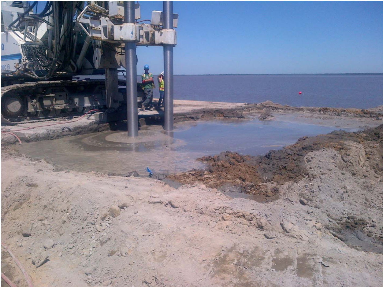
Figure 1.1 Double auger wet soil mixing system evidenced by pond of fluid grout formed in treatment area.
